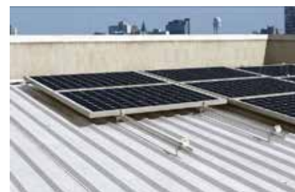
Industrial roof PV installation
